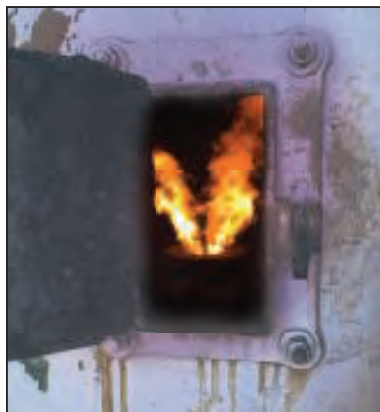
FIGURE 2. Faulty burner performance and improper flame-shape problems could not be solved by operators for a long period of operation time due to lack of troubleshooting knowledge
