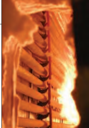
FIGURE 1. Faulty burner performance and continuous flame impingement have caused excessive tube-metal temperatures and coke buildup in heater tubes
