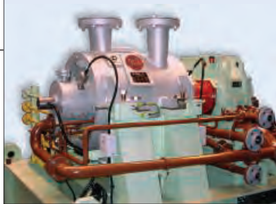
FIGURE 1. This centrifugal compressor is an electric-motor-driven machine that uses a gear unit for the speed match
